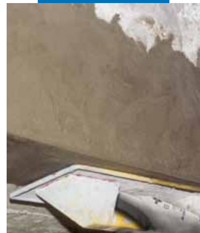
Patch-work of a concrete beam
